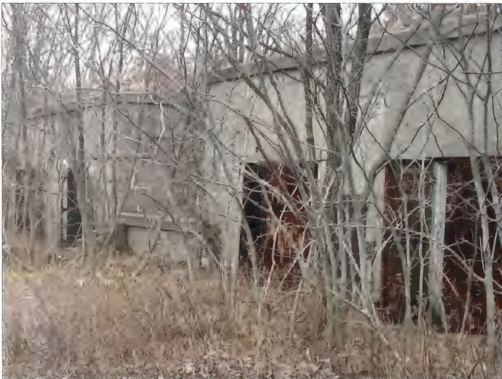
Figure 5.32. View looking northwest at south facade, Battery Morris. Accumulated leaf litter and debris should be removed from the front of the doors in order to remove a source of moisture that accelerates corrosion (Olmsted Center, January 2009).
